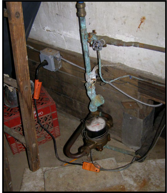
Water Meter, Water Main, Backflow Preventer
