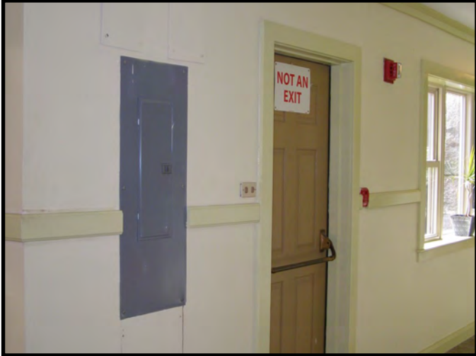
Electrical Panel - It's Salvageable or Replaceable. Planning Will Decide
