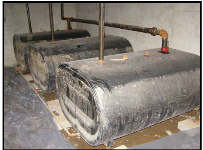
Oil Tanks - Located Below River Flood Level
