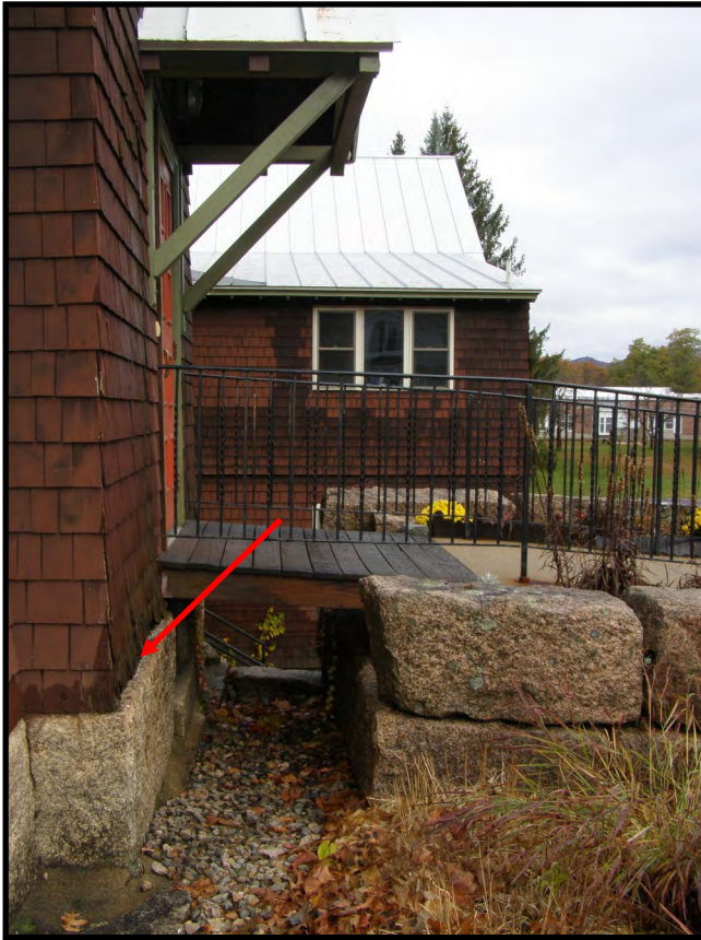
A Bad Original Building Detail - Rot Maker!
