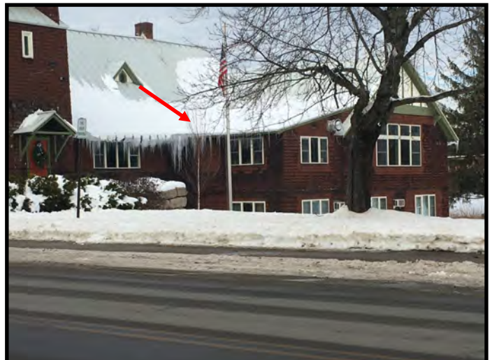
Ice dam and leaking roof valley
