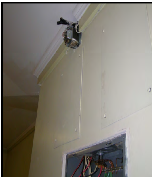
Mystery Transformer - LV Lighting Controls?
