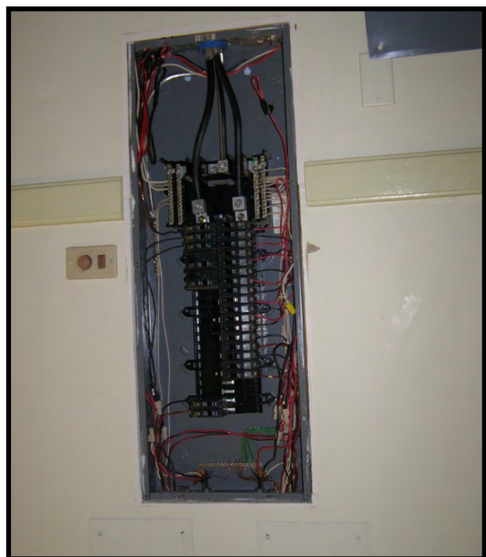
We Have Seen Much Worse Inside a Panel
