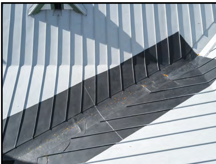
The Roof Valley "Repair" That Needs a Real Repair
