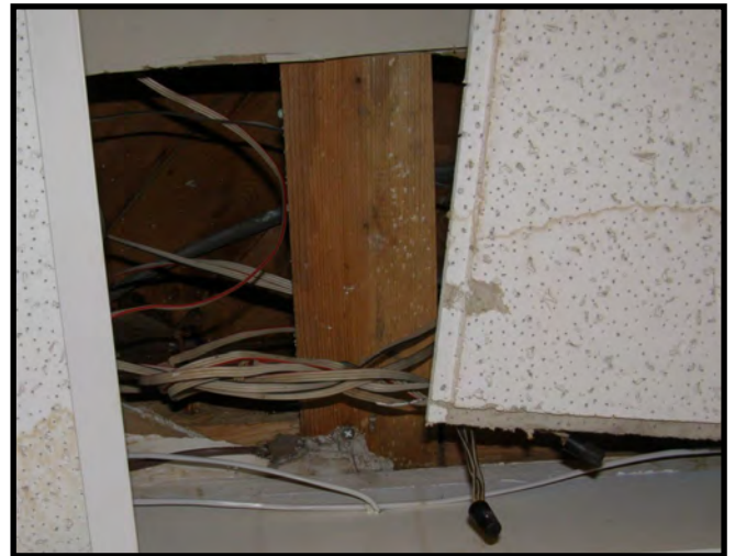
Electrical Clean-Up Is Necessary - Bell Tower
