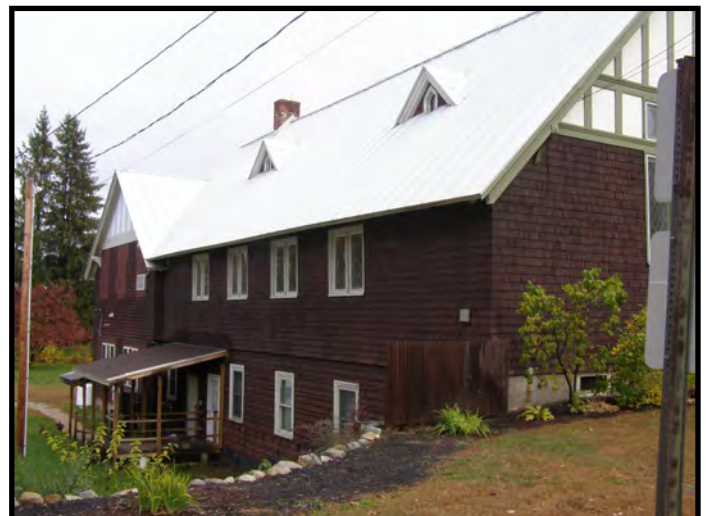
West Bldg Corner Looking North - Sanctuary Wall Badly Splayed
