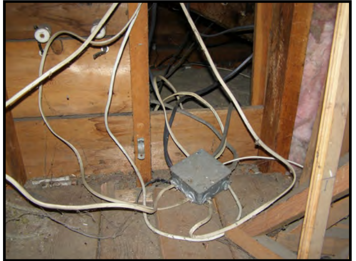
Electrical Clean-Up Is Necessary - Bell Tower
