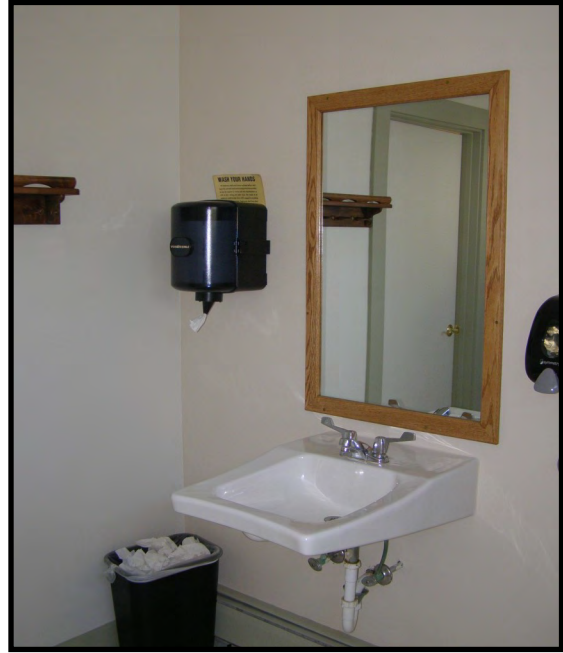
Fellowship Hall Restroom - Completely Salvageable
