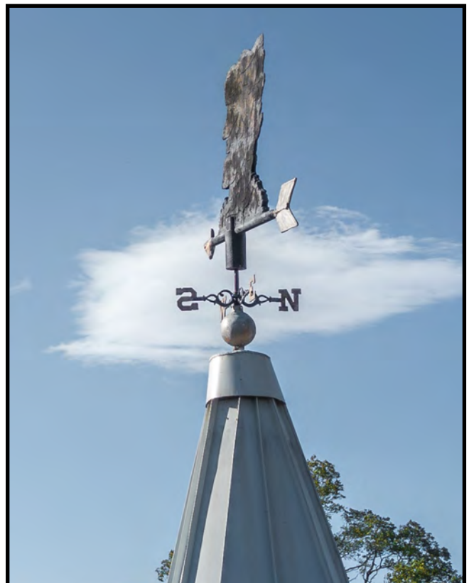
He Needs to Be Removed and Fully Re-Furbished
