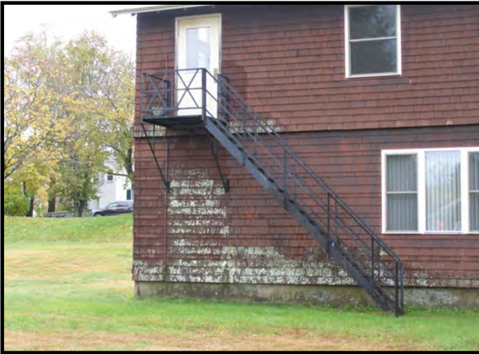
Fire Escape & Deteriorated Siding - Time to Replace Both
