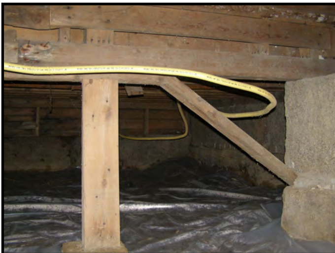
A Horribly Non-Compliant Propane Pipe Installation
