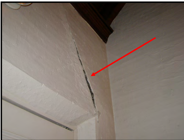
Deteriorating Sanctuary Plaster Is a Serious Concern
