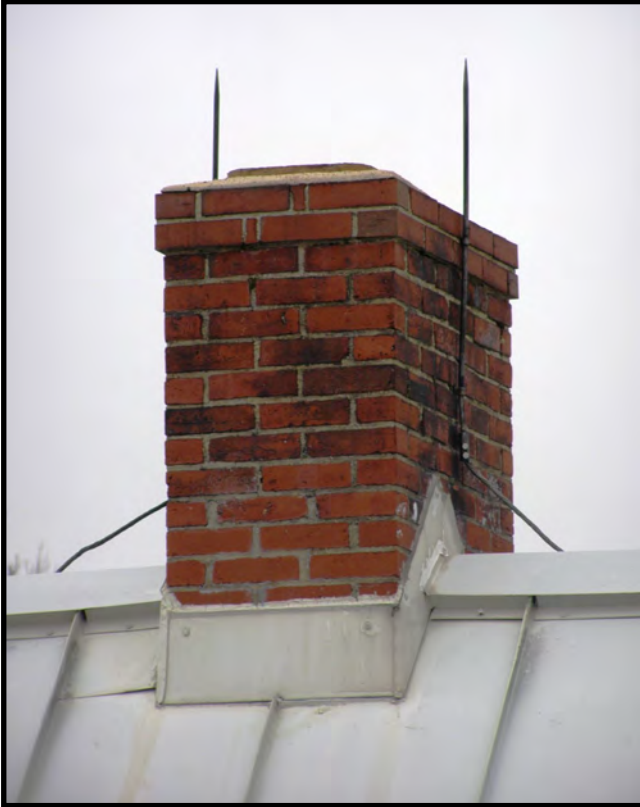
The Chimney - Let's Make It Go Away
