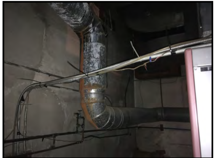
Furnace Vent Connector - Must Be Corrected
