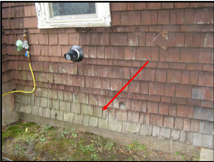
Red Arrow Indicates More Water/Rot Deteriorated Siding
