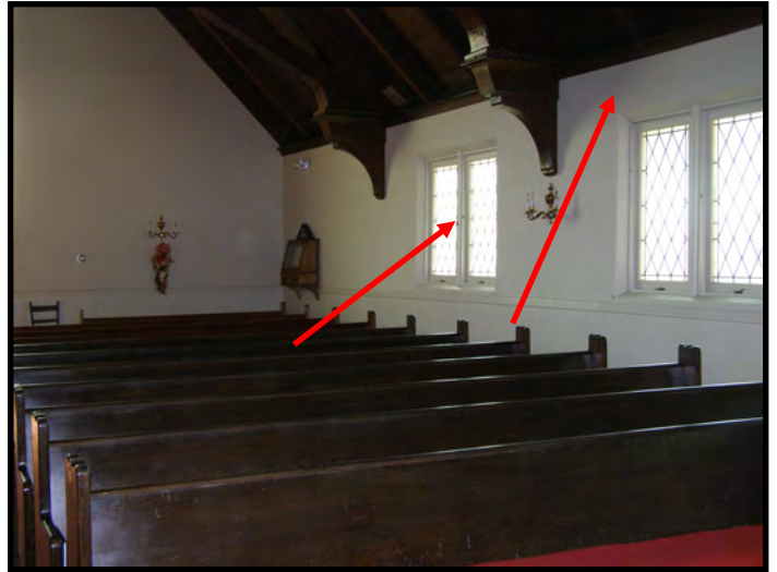
West Sanctuary Wall. Arrows Indicate Where Wall Is Tipped Outward and Stain-Glass Windows That Need Preservation
