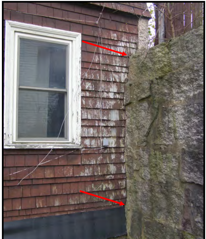
Arrows Indicates Rot - Lower Arrow Indicates Opening Into the Building. South West Corner of Building
