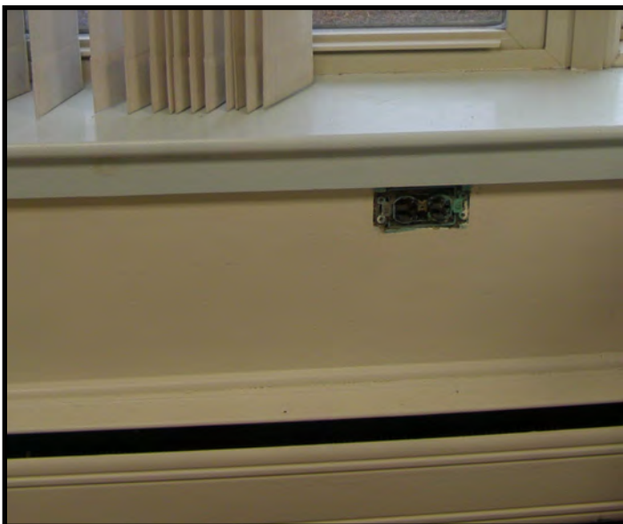
Electrical Clean-Up Is Necessary - Lower Level Meeting Room
