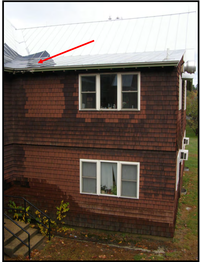
An Example of How to NOT Do a Roof Valley
