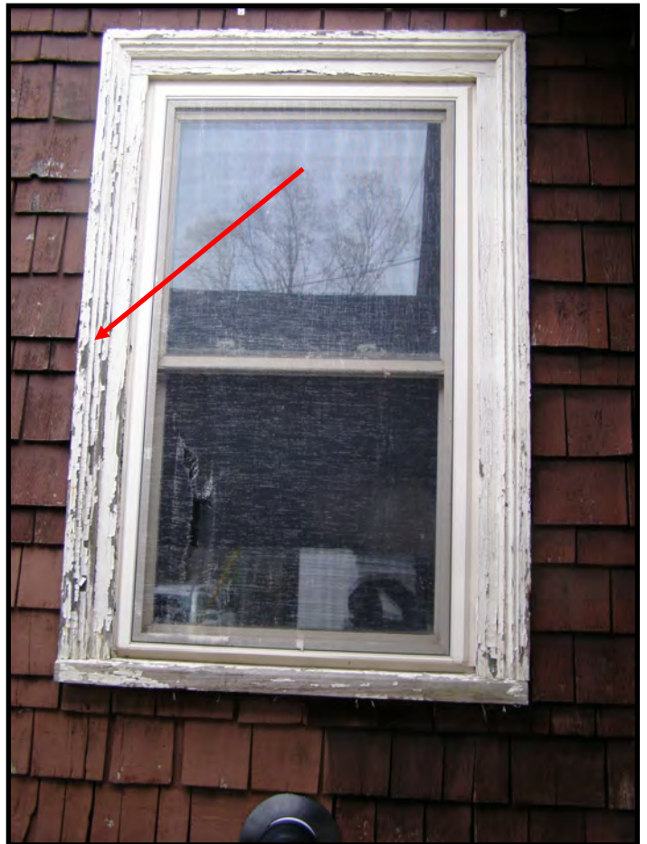
Replacement Window in Original Frame. Arrow Indicates Flaking Lead Based Paint
