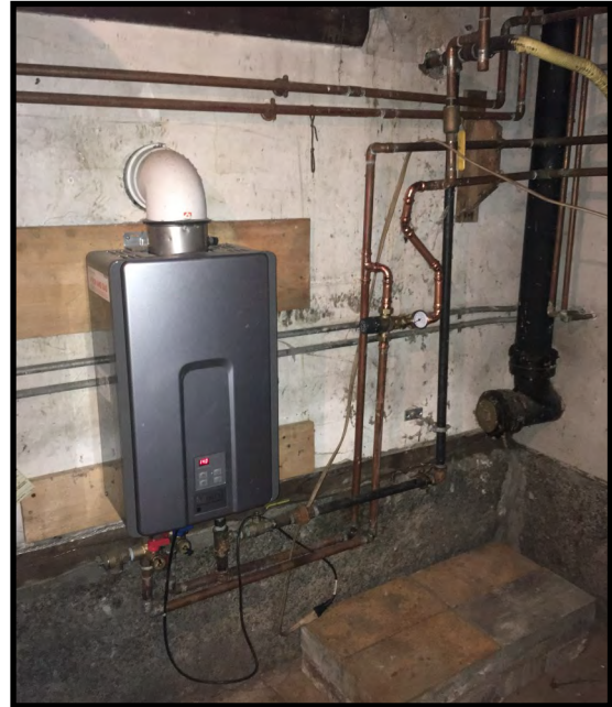
A Good Water Heater - Improve Installation
