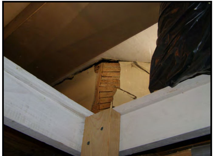
Lower Level South Exterior Wall - Plaster Deterioration as Wall Dropped, Due to Floor Having Dropped Out Beneath the Wall
