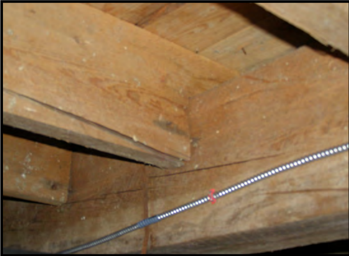
Proper Wiring Method & Improperly Notched Floor Joists
