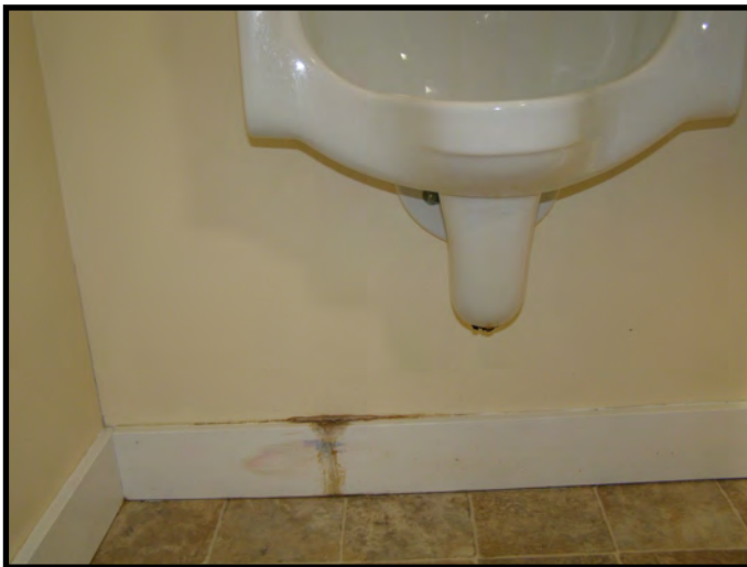
Mens Room - Active Leak?
