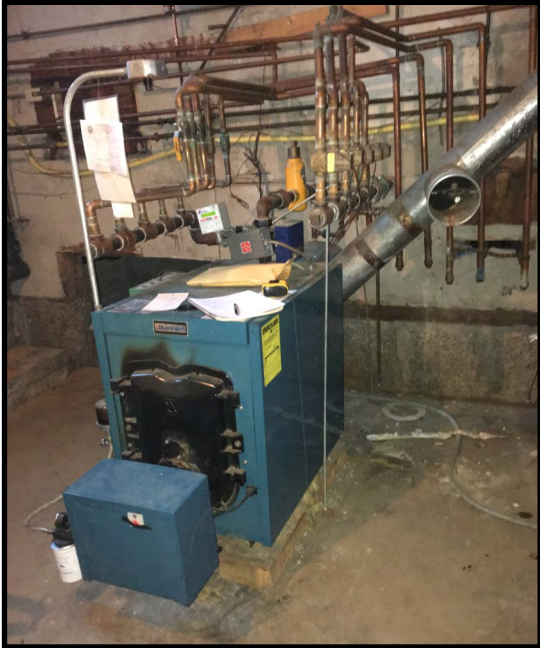
2007 Boiler - Needs Maintenance or... Replace?
