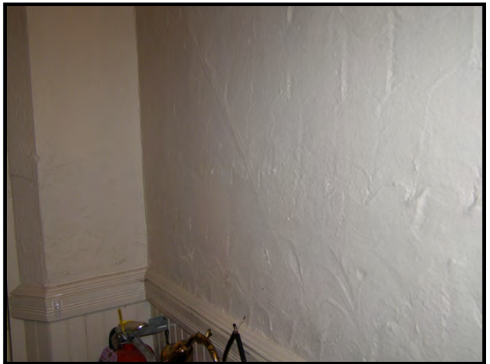
Deteriorating Sanctuary Plaster Is a Serious Concern
