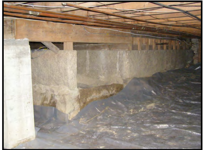
Transition Original to 1955 Foundation In 1955 Crawlspace. Granite Wall is North End of Original Building
