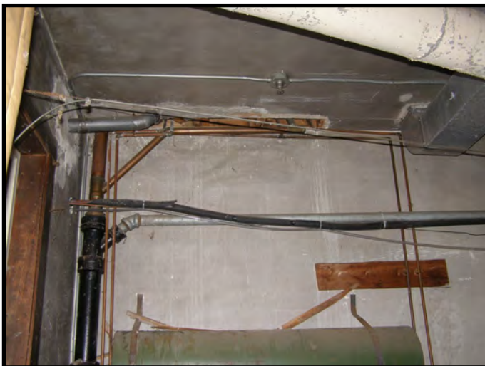
Mechanical Room Plaster - More Asbestos to Address
