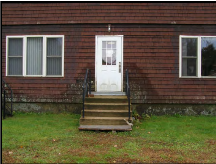
Lower Hallway Exit Towards the North - Note Siding Condition
