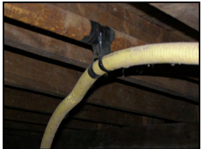
The Same Horribly Non-Compliant Propane Pipe Installation
