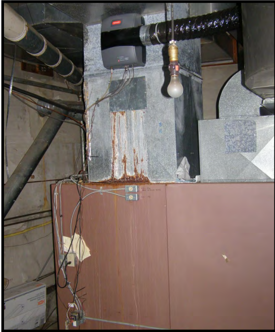
The Furnace Is Nearing End of Life
