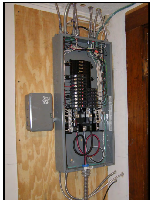
Nicely Installed "New" Electric Panel
