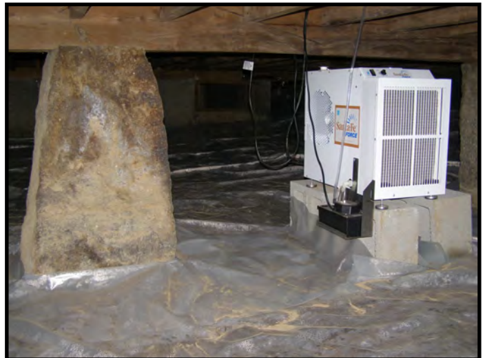
Dehumidifier Beneath Food Pantry - Nicely Done
