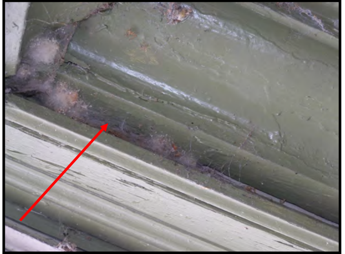
This Appears to Be Fiberglass Insulation Which Is NOT an Original Building Component
