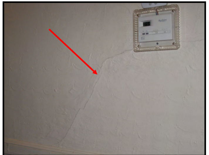
Deteriorating Sanctuary Plaster Is a Serious Concern
