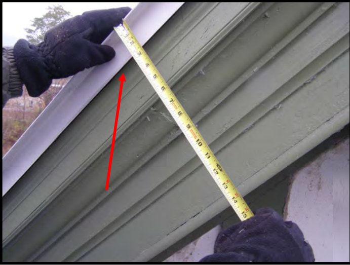
Red Arrow Indicates an "Out of Place" Molding That We Believe is Concealing Insulation of Some Type
